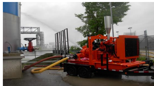
Testing of emergency mitigating equipment at the Darlington Nuclear Generating Station.
