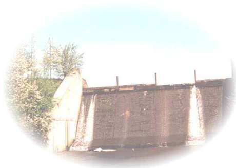
Figure 49 Spillway at McLaughlin Road Reservoir. At left are Pin Cherry trees in blossom.
