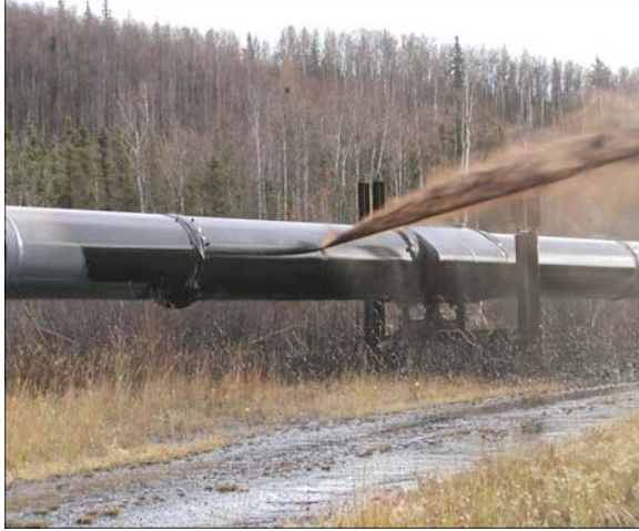
Figure 10. An intentional breach of an Alaskan pipeline.
