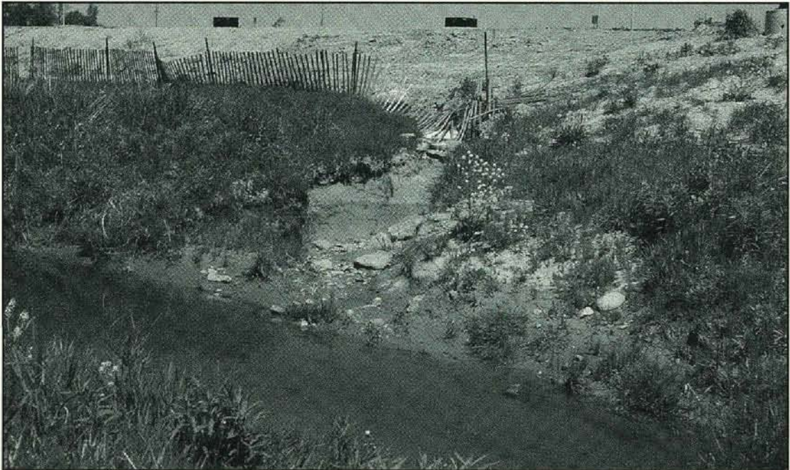
Careless site preparation damages soils, watercourses, and wildlife habitats
