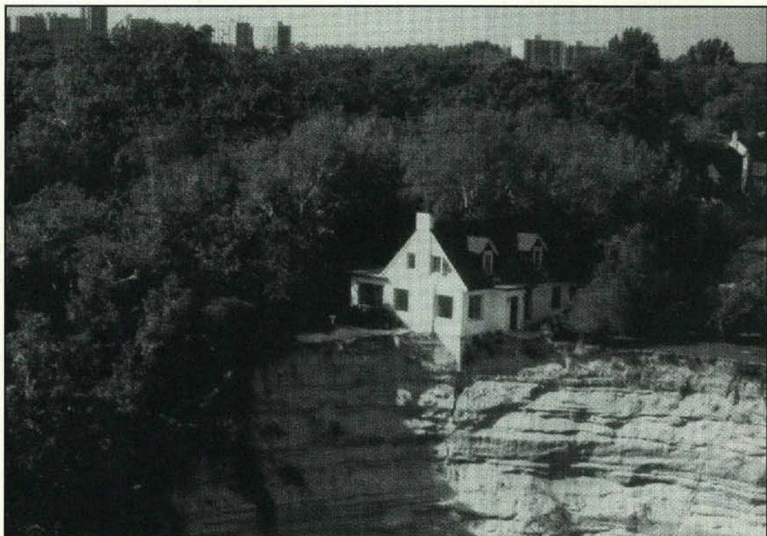
House atop eroded Scarborough Bluffs
