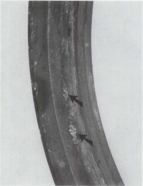
PHOTO 10 Porthole No. 4 showing impact marks and gouges (arrows) on the outboard edges of the porthole.
