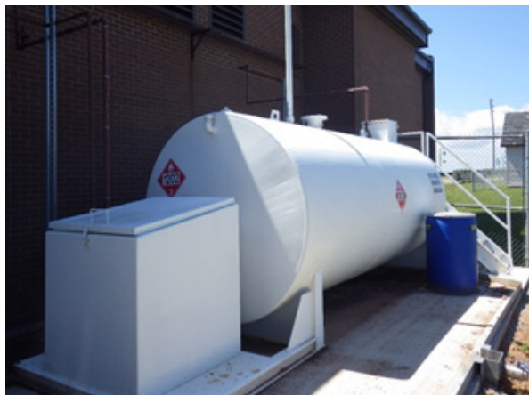
Diesel fuel tanks on First Nations are regulated under the Storage Tank Systems for Petroleum Products and Allied Petroleum Products Regulations. Photo: Fernand Comeau © Environment and Climate Change Canada
