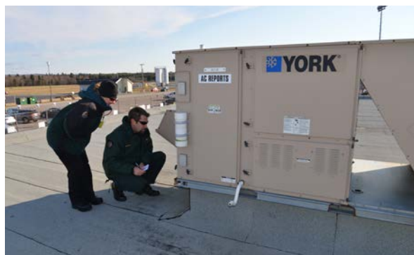
EC Inspectors check air conditioning units. Photo: Robert Robichaud © Environment and Climate Change Canada
