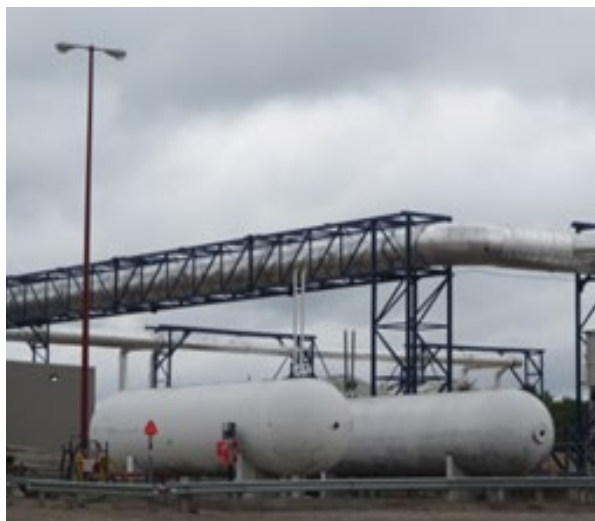
Propane storage facility regulated by the E2 Regulations. Photo: Gerard Chisholm © Environment and Climate Change Canada
