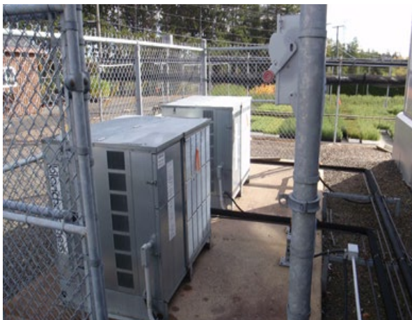
Air-conditioning units fall under a new Code of Practice designed to reduce and prevent emissions of halocarbons into the environment. Photo: Fernand Comeau © Environment and Climate Change Canada
