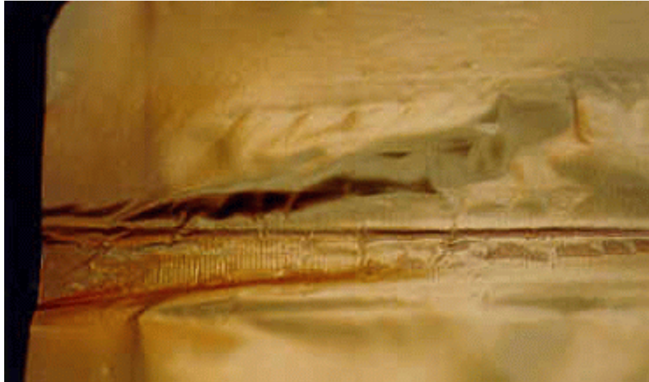
Delamination and Bubbling of the Polyester Laminate
